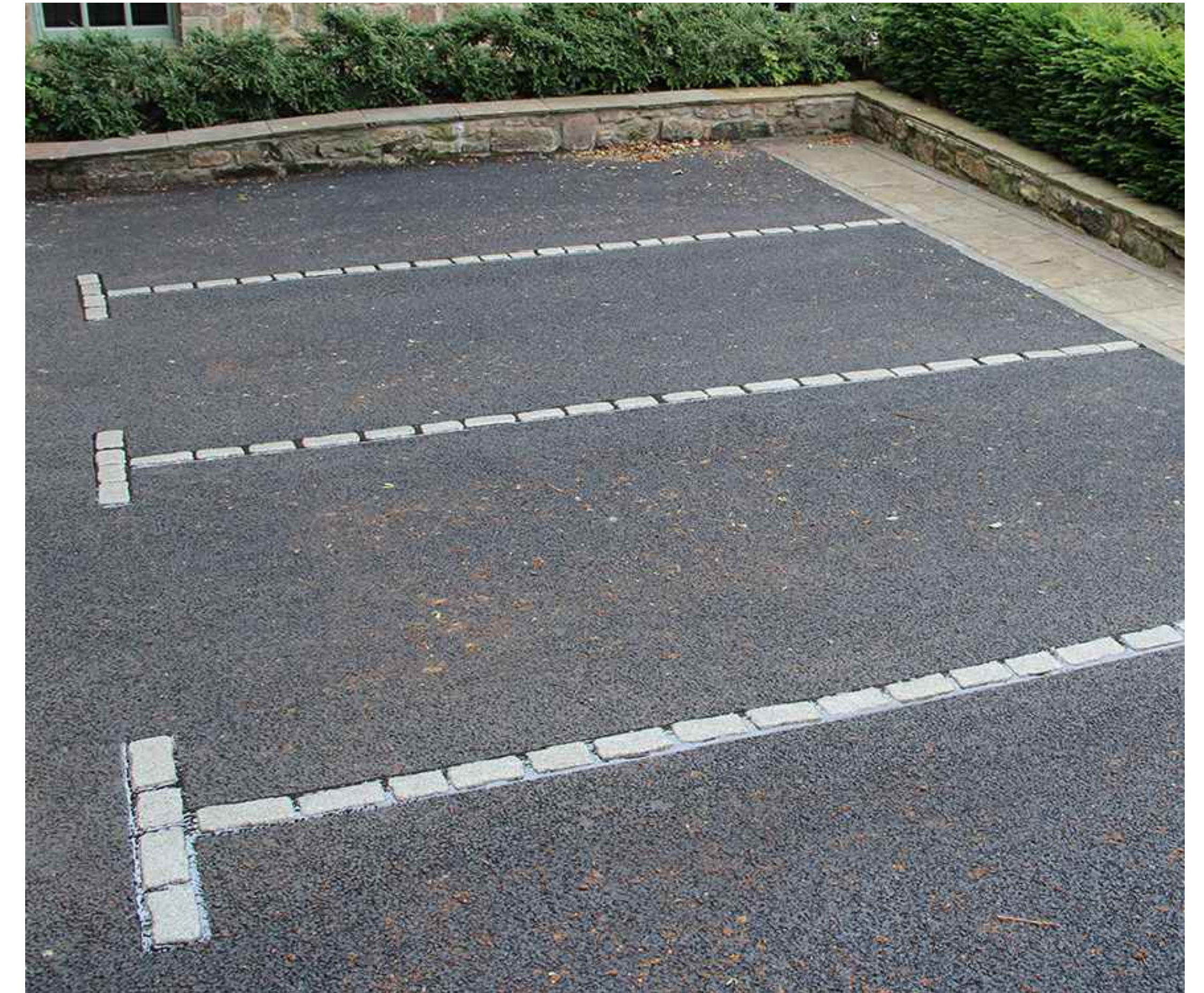
COBBLE SET IN CONCRETE (PARKING SPACE DELINEATION) (SEE PLAN FOR LOCATION/LAYOUT) NOT TO SCALE
